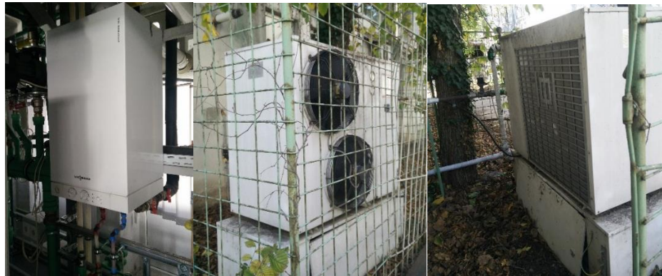
Fig. 31– The equipment (boiler and chiller) that heats or cools the climatic chamber
