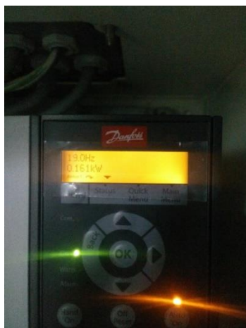
Fig. 39 – The VLT HVAC Basic Drive at 19.0Hz
