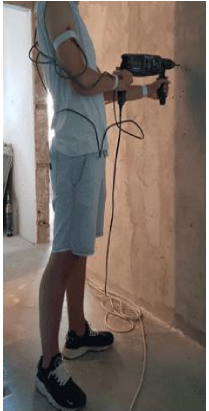
Fig. 4.11. Percussion drill mounted data collection system - side view
