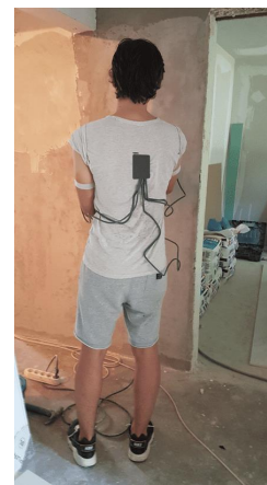
Fig. 5.8. Mounted acquisition system for percussion drill data collection - rear view
