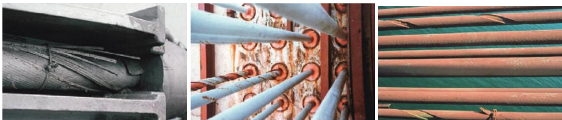
Figure 2 – Cable stays degradations
