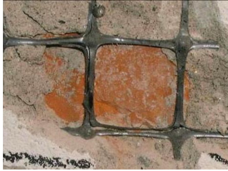
Fig. 5.4.6. The solid brick model – the bricks are still intact, while the reinforcement broke down [47]
