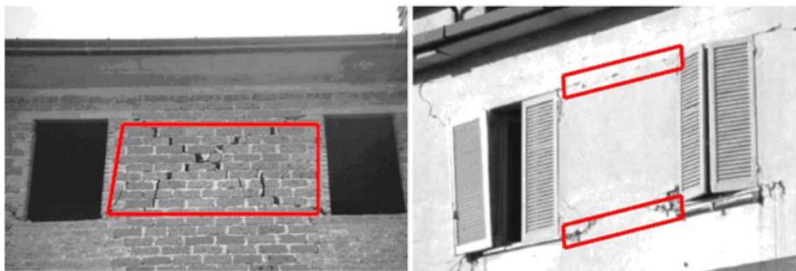
Fig. 5 Damage patterns observed after the earthquake for masonry structures (S.T.A. DATA 2012)
