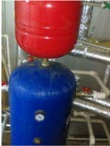
Figure 43 Experimental study bench heating accumulator with expansion pressure tank
