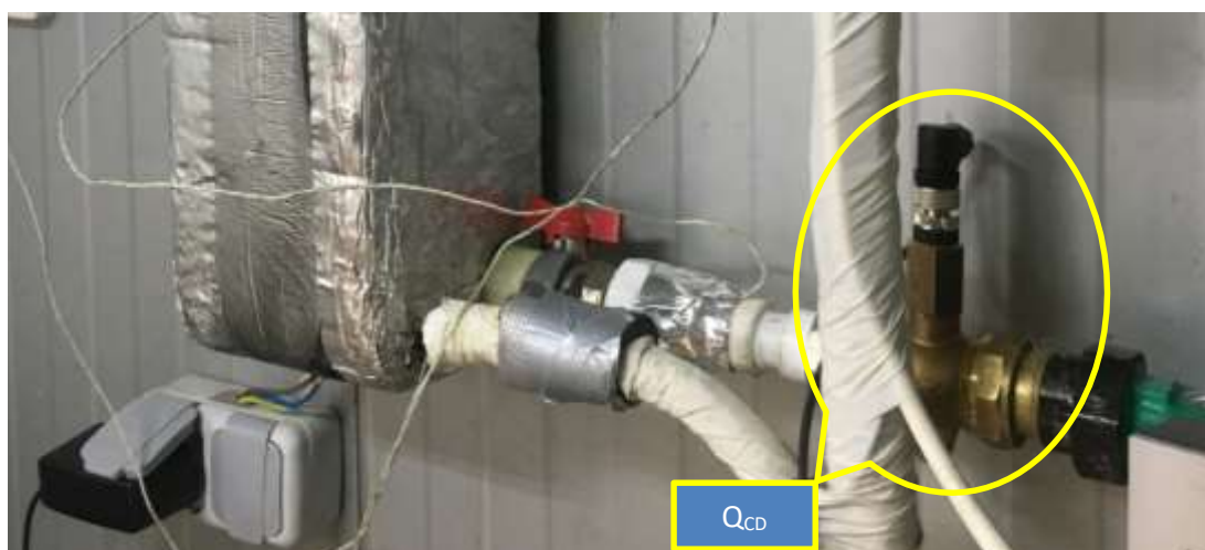
Figure 52 Experimental study bench flowmeter installation
