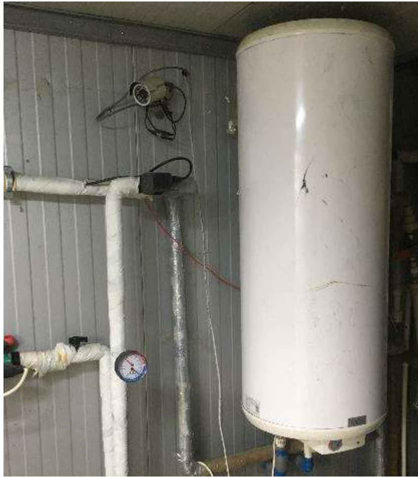
Figure 42 Experimental study bench DHW water tank and three way selection valve.
