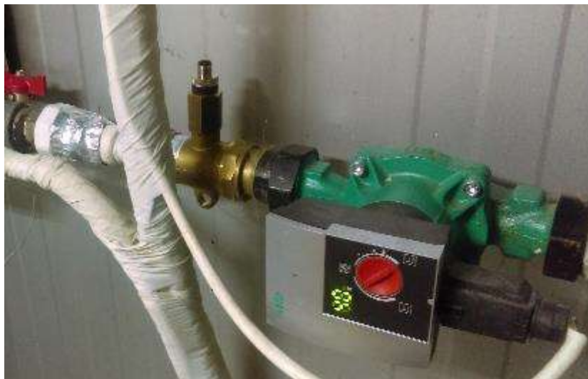
Figure 46 Experimental study bench condenser secondary line circulating pump
