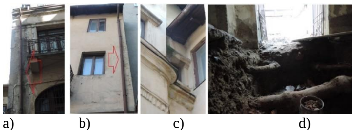
Figure 6.25 - a) Degradation of exterior plasters, caused by damaged rainwater collection and management systems; b), c) Traces of rainwater infiltration; d) Obsolete sewerage installations [122]
