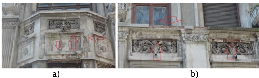
Figure 6.24 - a), b) Degradation of the main facade plasters [122]
