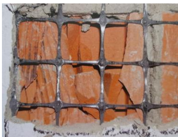
Figure 7.7. Degradation of bricks with gaps
