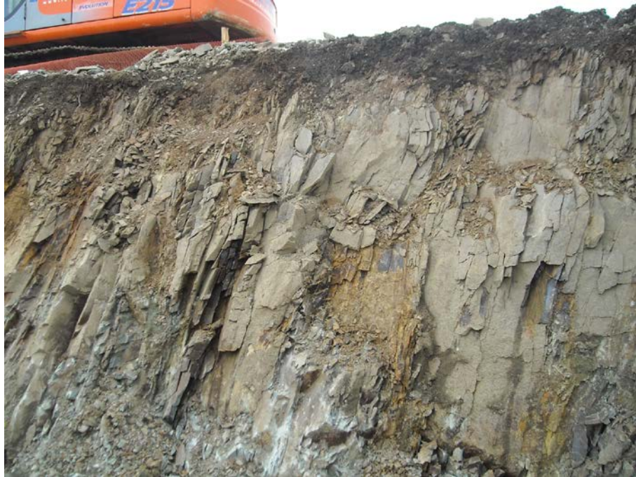
Figure 21. Rock cracking state - green schist- in the Dobrogea area
