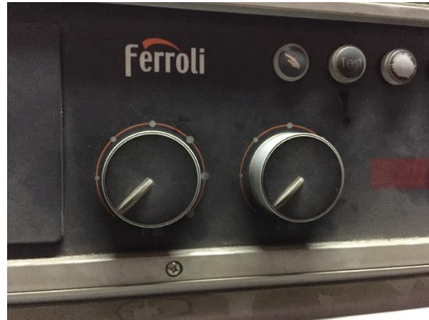
Fig.29 a)Operating conditions b)control panel of the boiler T1-stage1 / T2-stage2
