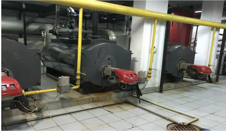
Fig.26 Central heating on the inside
