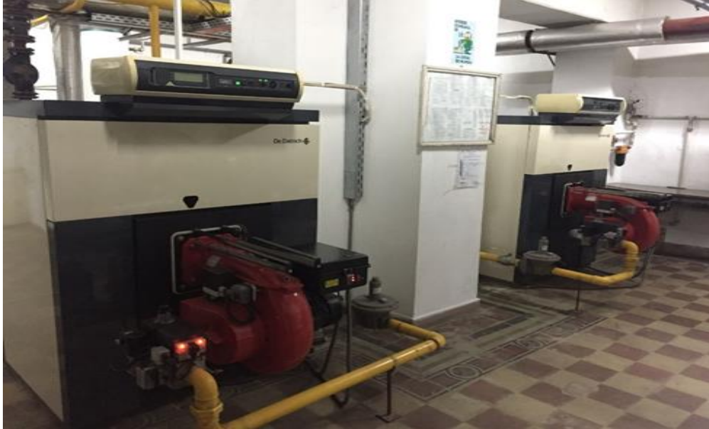
Fig.37 Central heating on the inside
