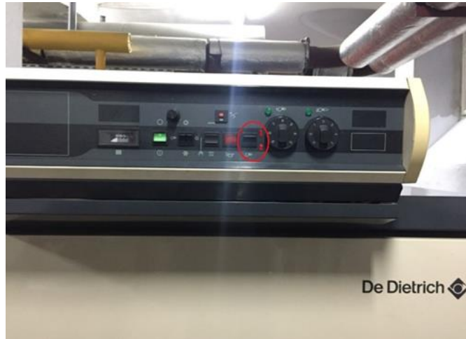
Fig.40 a)Operating conditions b)control panel of the boiler T1-stage1 / T2-stage2
