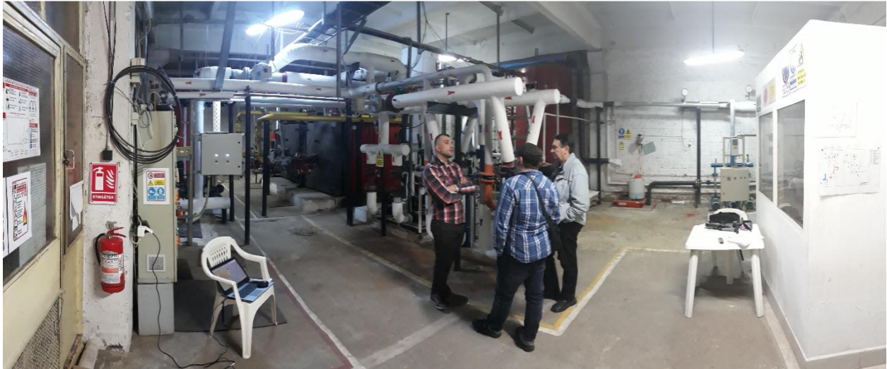
Fig. 8 Boiler plant on the inside
