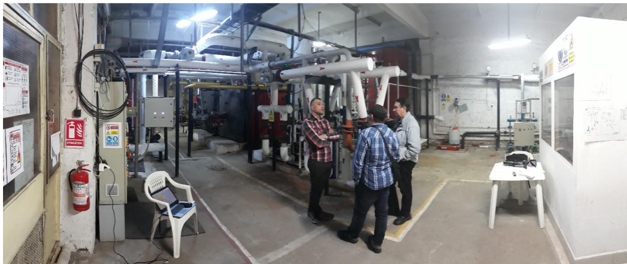
Fig. 8 Camera centralei la interior
