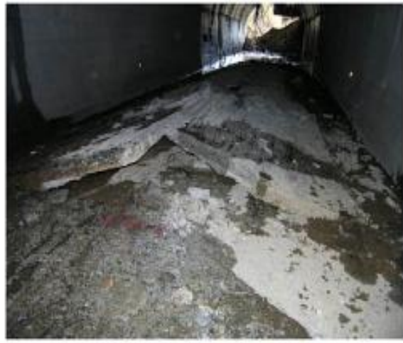
Fig.4.9. Exfoliations of the coating in the Haguro tunnel
