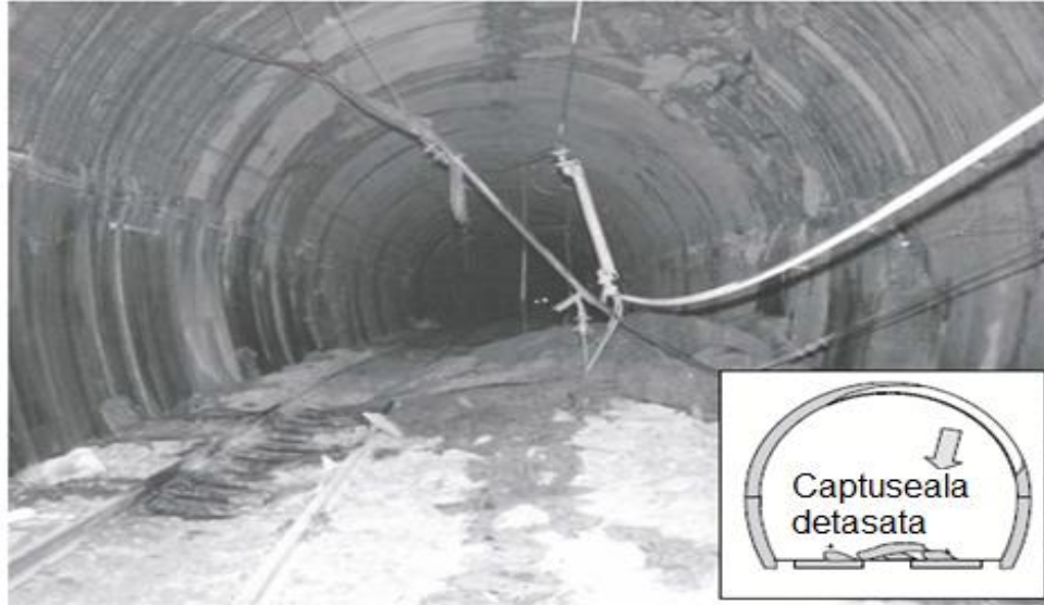
Fig.3.18 Damage to the Wanatsu tunnel
