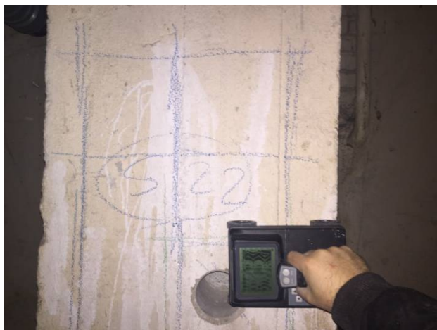
fig.2.2.relevu structura vericala beton armat (stalpi) realizat cu GEORADAR GSSI-1GHZ
